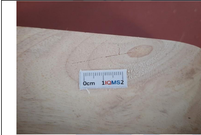
Crack on Surface
