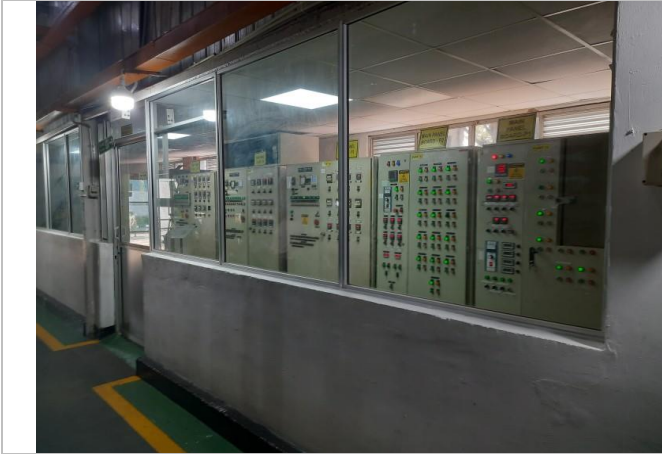
Main Panel board Area
